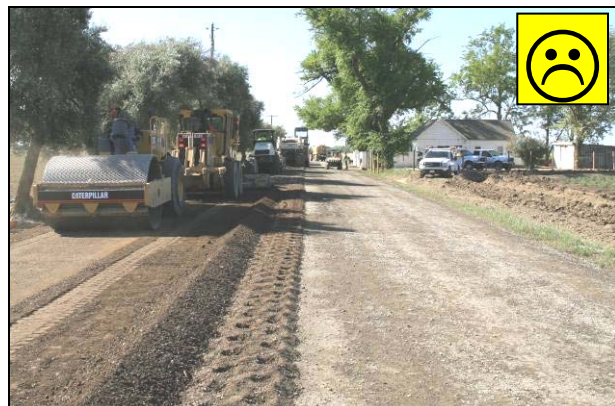
Figure 6.42: Final leveling and compaction interfering with initial compaction.
